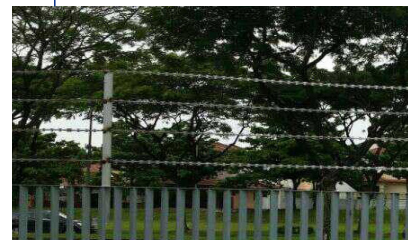
For road perimeter protection
